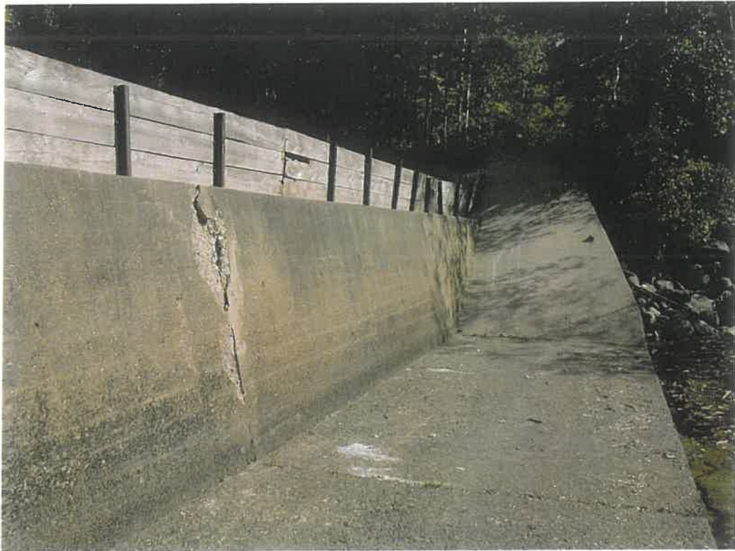
Photo 1 – Concrete deterioration at construction joint
