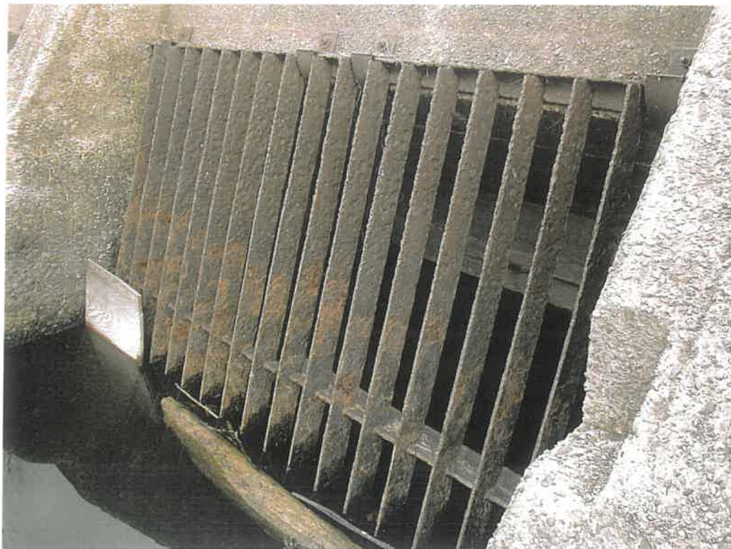
Photo 4 – Trash rack pitting
