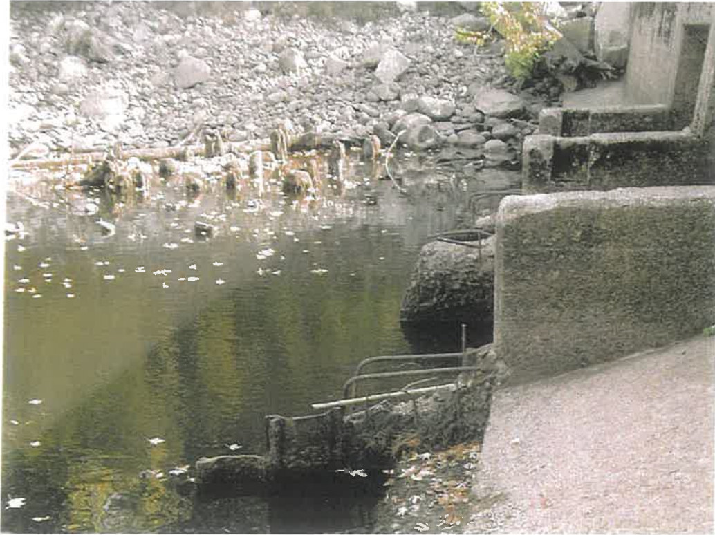
Photo 3 – Concrete gate pier deterioration
